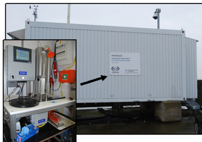
Figure 1: Picture of the automated filtration module installed in combination with the FerryBox system in the COSYNA container in Cuxhaven.
